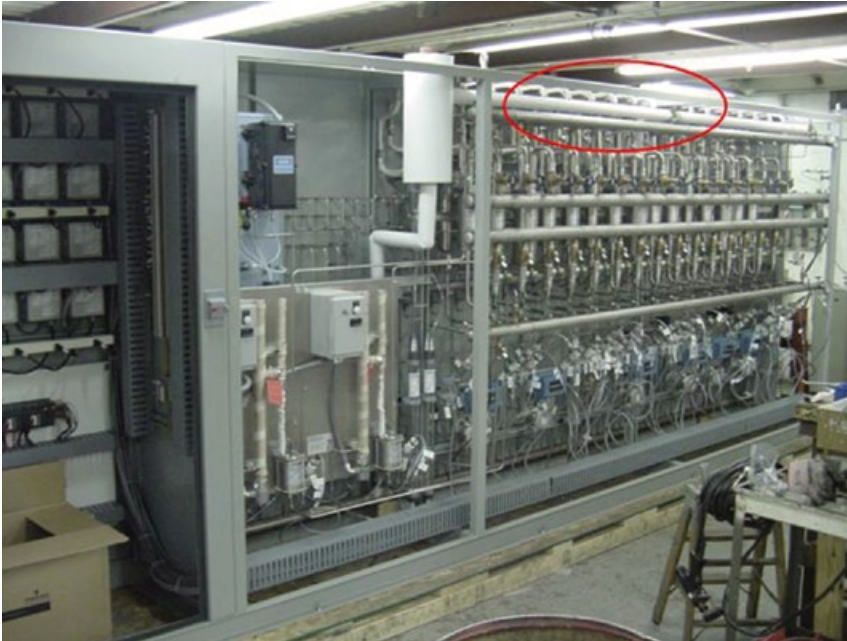
3. Blowdown lines at top of panel are provided to flush sample lines at the beginning of each startup
